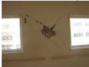
Photo 2. Damage of column (damage level ) of 2nd floor (TS-1 building of TS-High school)
